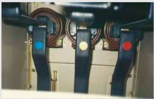
Bus bar insulating covering (NPN)
