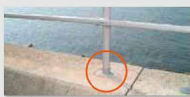
Corrosion prevention of coastal guard rail ground-contact points (NOR-A)
