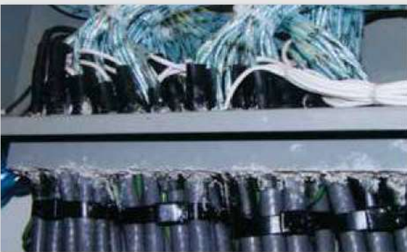
Control panel cable bundling (NOR / NON)
